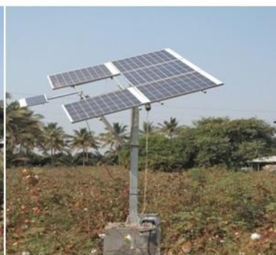
Fig 2 Designed Solar PV system installed at site
