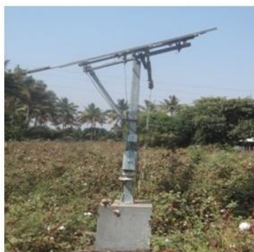
Fig 1 Side view of installed solar PV system
